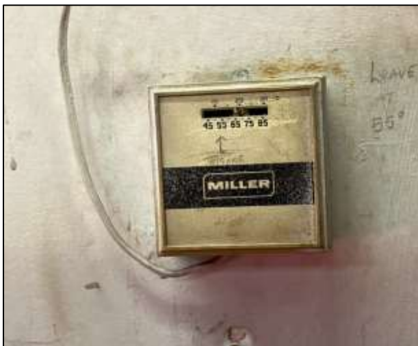
Existing thermostat in apparatus bay
